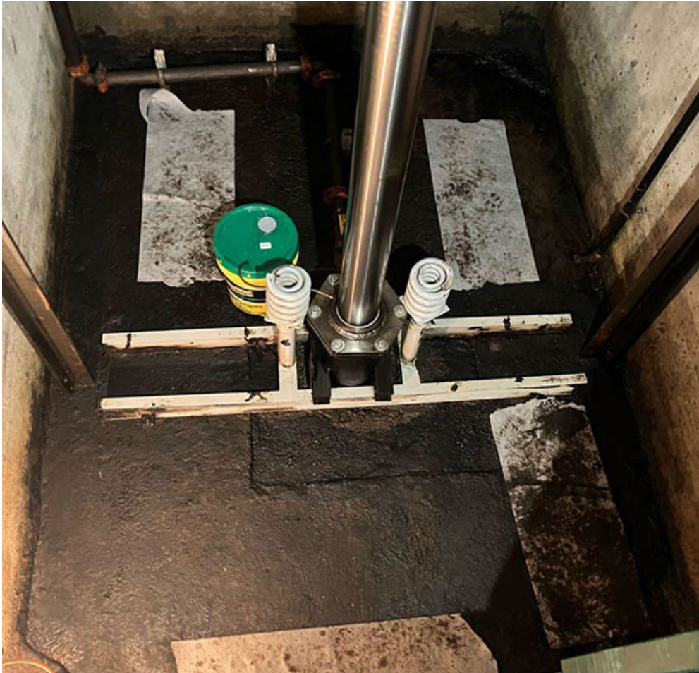
Tar revealed at the bottom of the pressure washed pit
