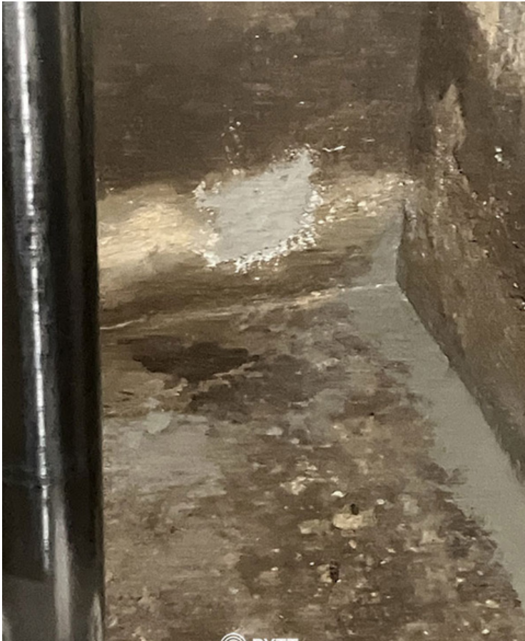
Back wall void, right side
