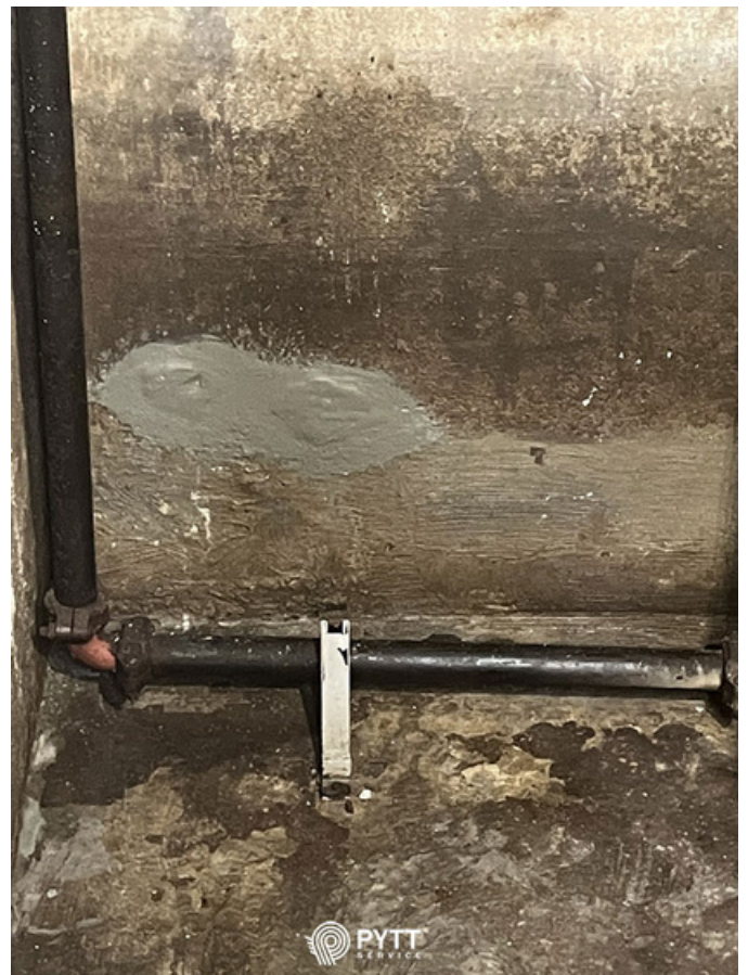
Back wall void, left side
