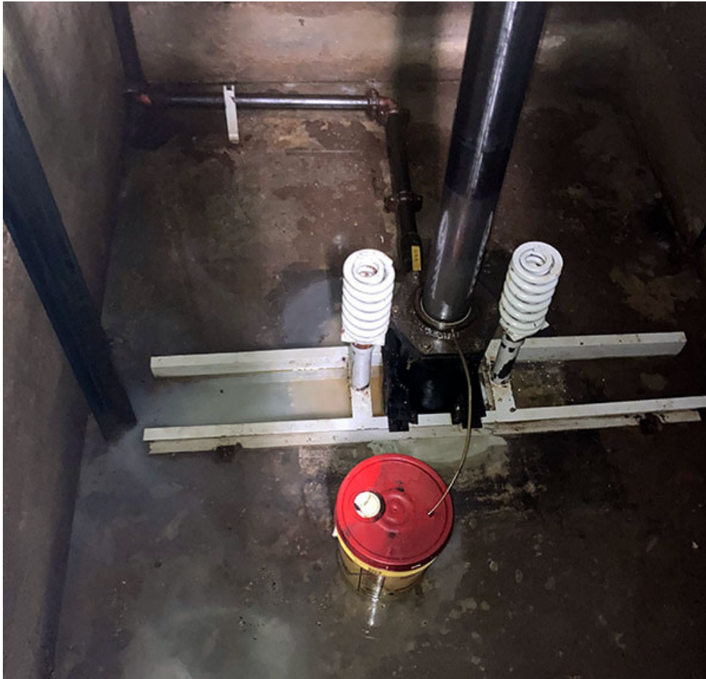
After rain test - approx. 2 inches of water
