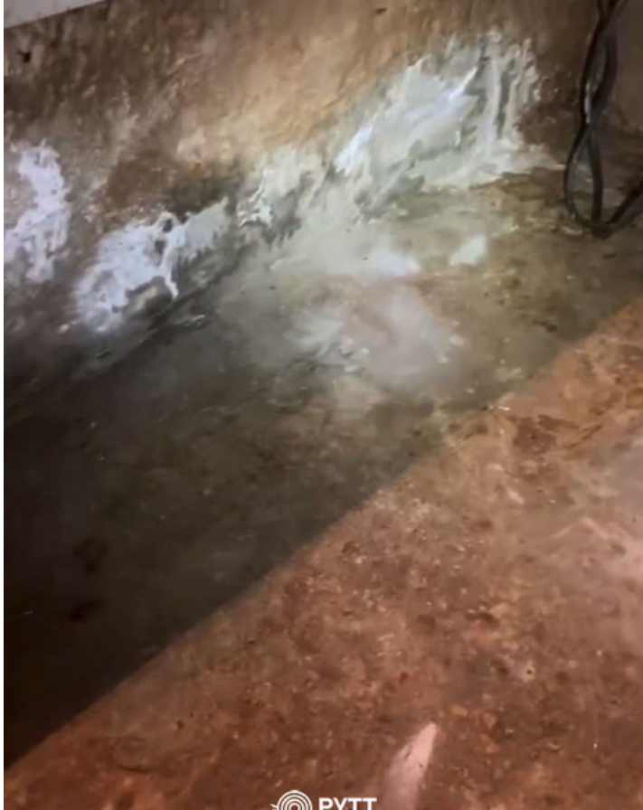
Door-side water intrusion (L)
