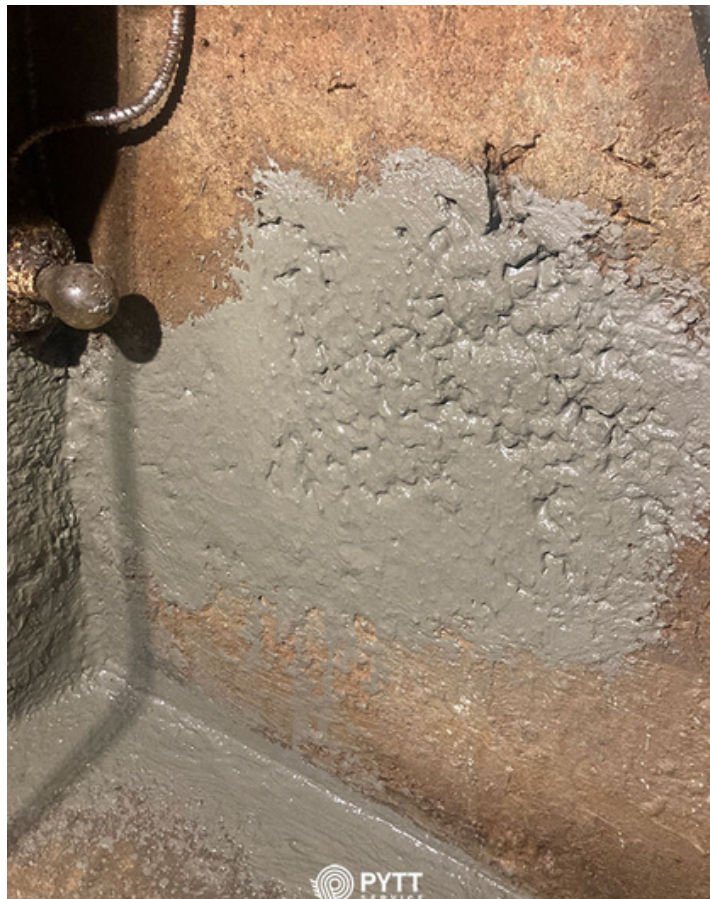
Honeycombed wall waterproofed
