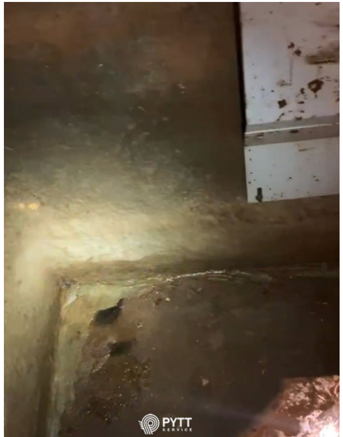
Door-side water intrusion (R)
