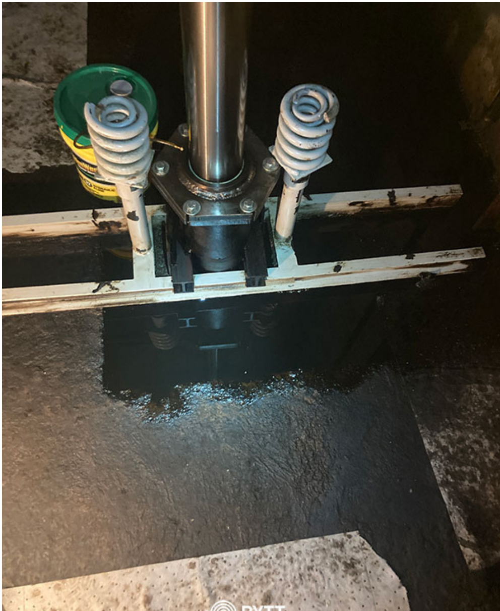
Rising water levels revealed oil from the jack casing
